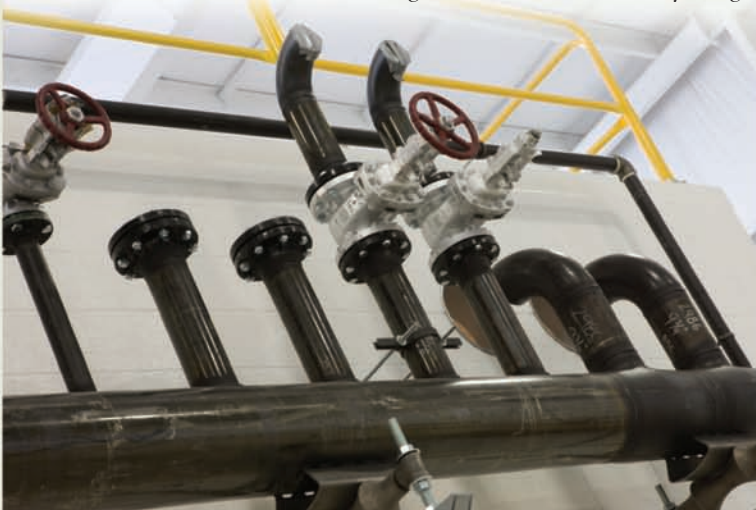
Kline's Services' food-to-fuel conversion system is one of only four that have been designed and installed nationally. The building housing the system was built with the help of an SBF loan facilitated by EDC Finance Corporation.
